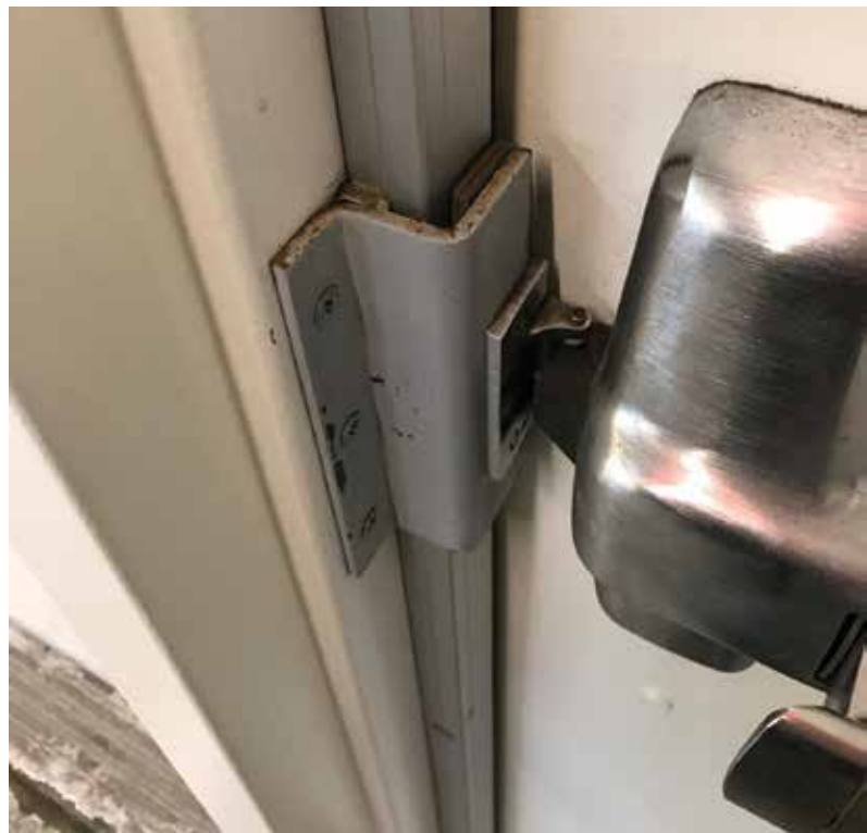
Figure 3: The proper way to install a security bracket to allow for a surface mounted roller strike to be installed.
