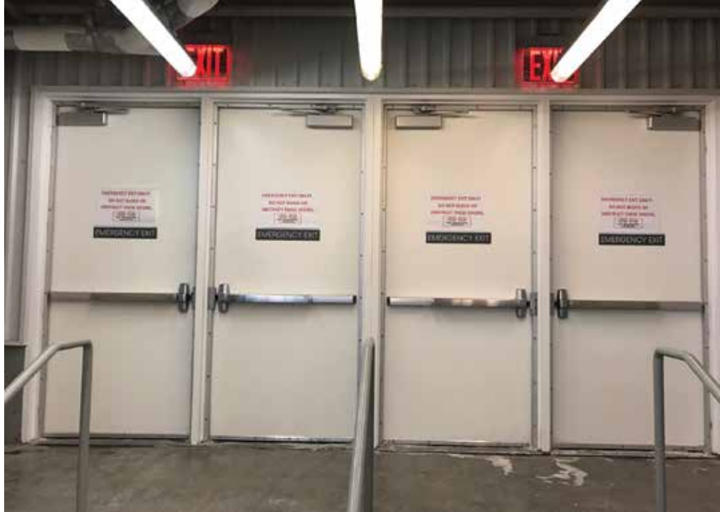
Figure 2: A good representation of how hardware should be mounted to gasketing in a school application.
