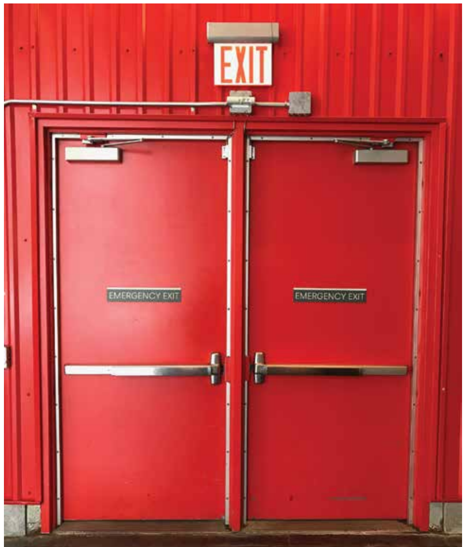
Figure 1: The mounting hardware used for the door closer and strike has been properly specified and installed.
