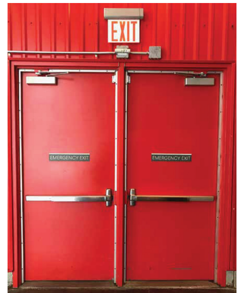
#5077 installed in conjunction with #5077SPB.
