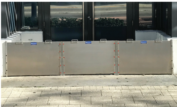
#5129MA mounted to front of hotel entrance.
